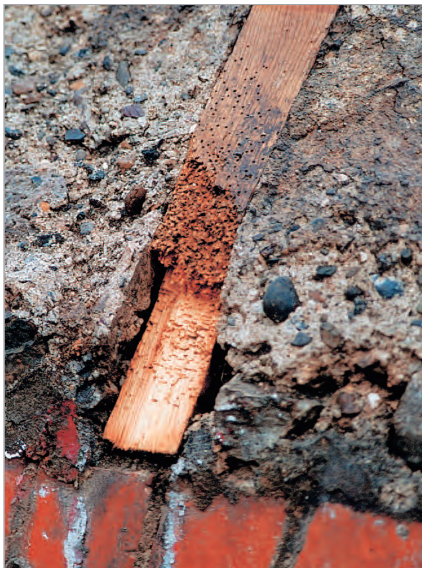
Woodworm infestation of roof rafter at eaves. High moisture content due to restricted ventilation.
