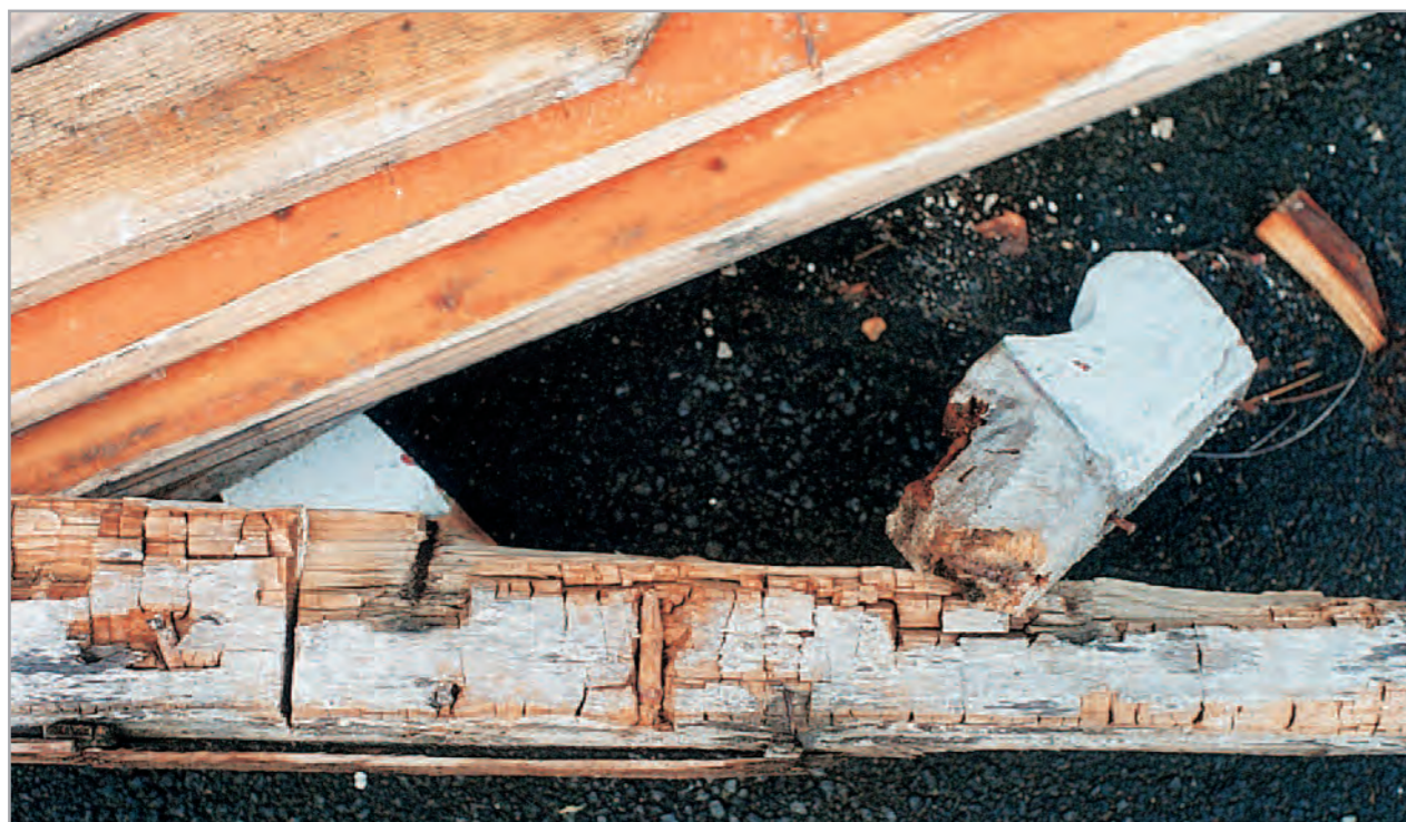
Dry rot damage to roof rafter caused by water and lack of ventilation.
